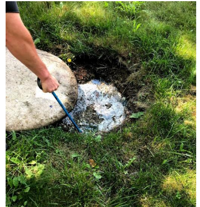
Failed Block Cesspool
