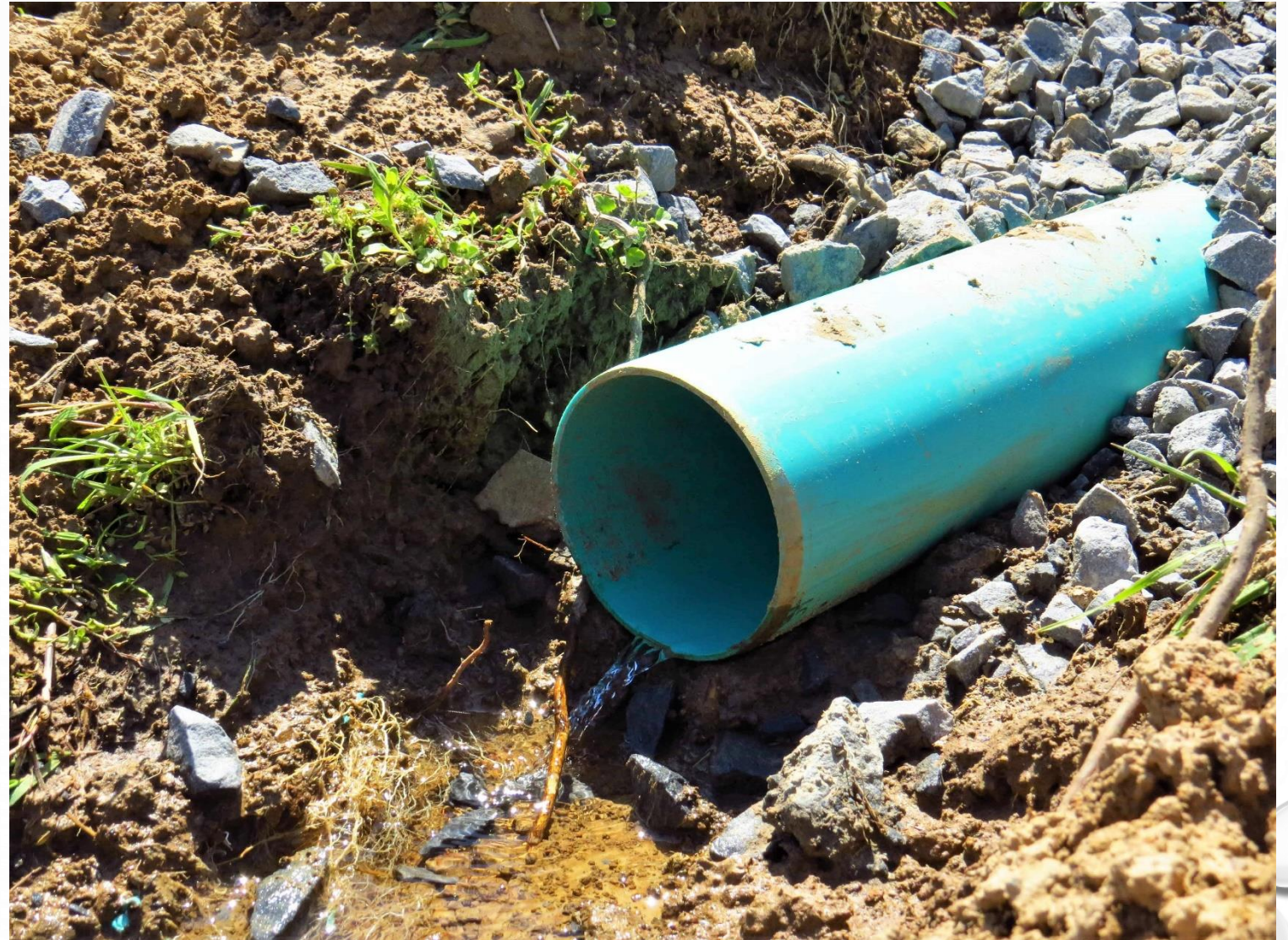
Surface Discharge – Round Mountain, Conway, Arkansas
