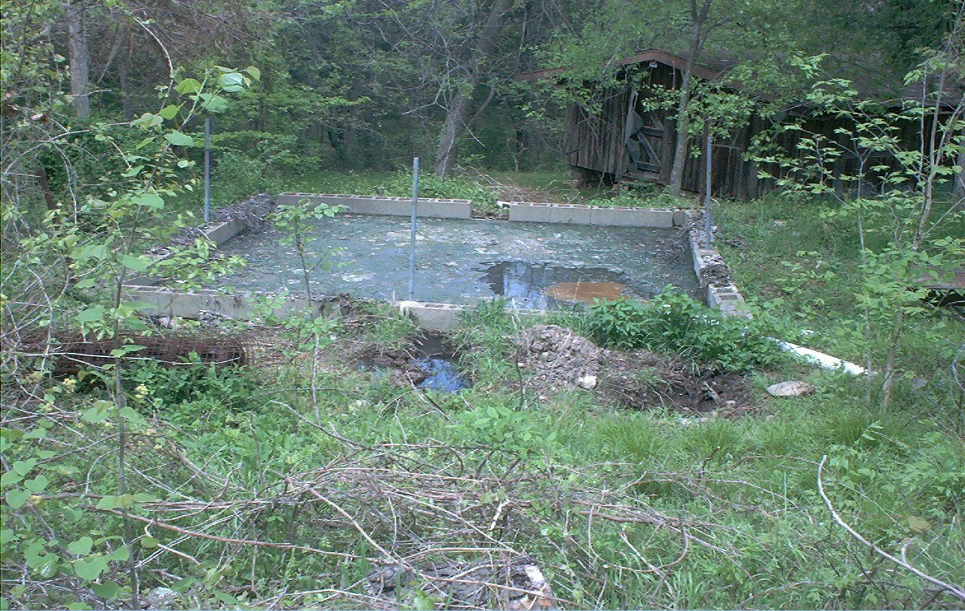
Single cell lagoon serving a small restaurant, restrooms, and owner's home.
