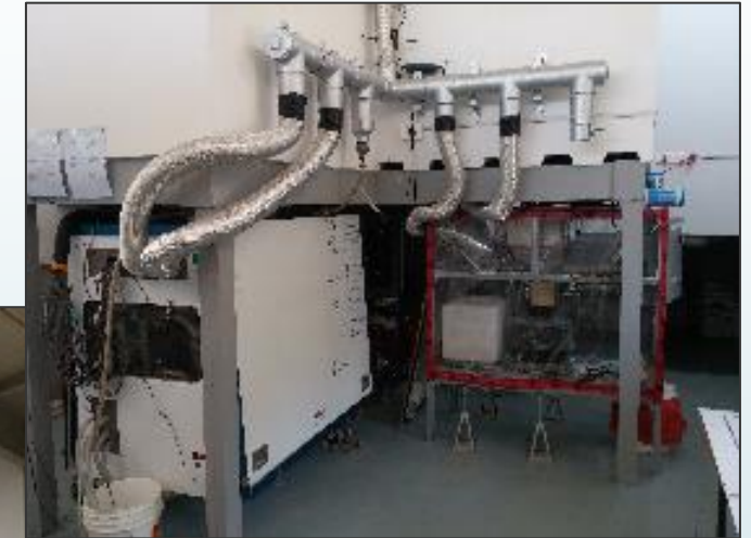
Engineering prototype installation in India in mid-2017.
