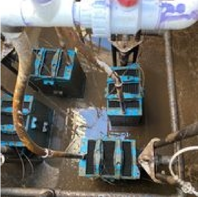
Figure 11. HSMBR after pumping out excess solids and cleaning in place
