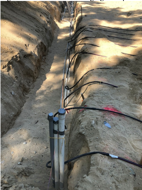
Figure 19. Geoflow ® drip line feeding header and footer installed below freeze depth
