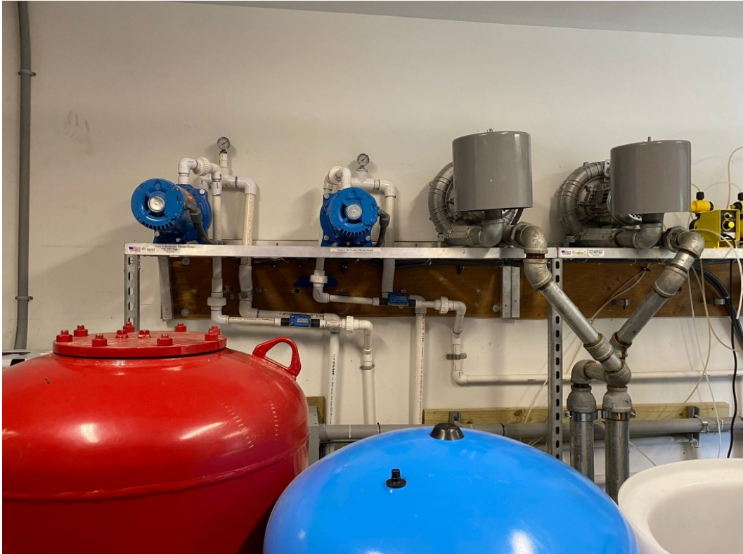
Figure 15. On wall inside sewage house 2 vacuum pumps, 2 linear blowers for coarse bubble diffusers
