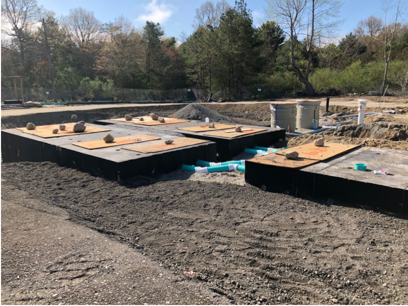
Figure 8. 10,000-gallon cast in-place tank (right) splits into two identical HSMBR treatment trains
