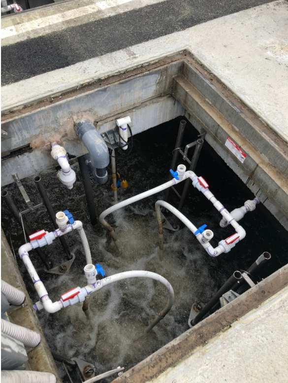
Figure 10. Coarse bubble aeration early in system operation
