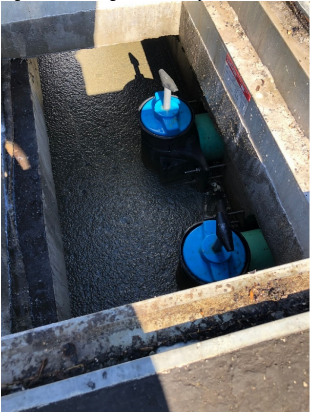
Figure 7. Two of four SaniTEE® effluent filters installed in 10,000-gallon cast in-place tank
