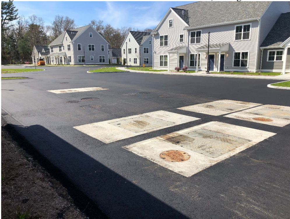
Figure 13. Installed tanks with access lids to grade, (foreground parallel treatment trains)
