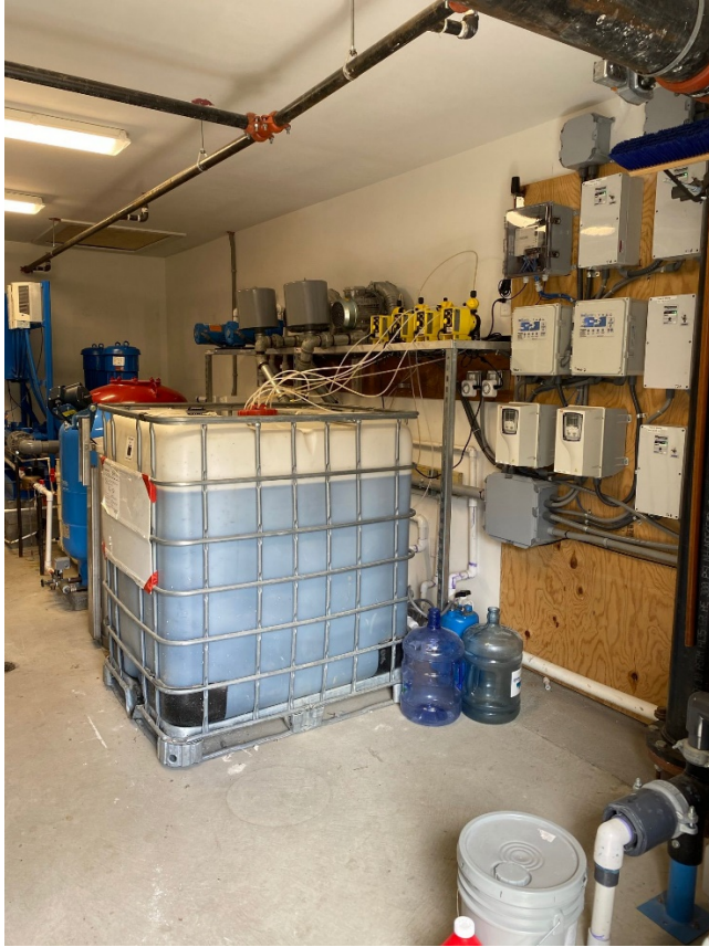
Figure 16. MicroC ® supply delivered by yellow chemical feed pumps on wall
