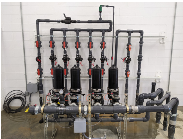
Photo 2. Filter and control options for a large drip system
