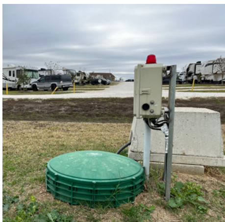
Photo 7. Monitoring an aerobic treatment unit at a Texas RV park.
