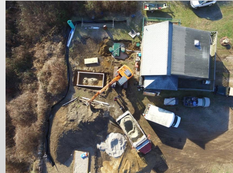
A Nitrogen reducing OWTS is installed to replace a failing metal tank system located less than 100 feet from a coastal wetland under the Charlestown EPA SNEP Grant
