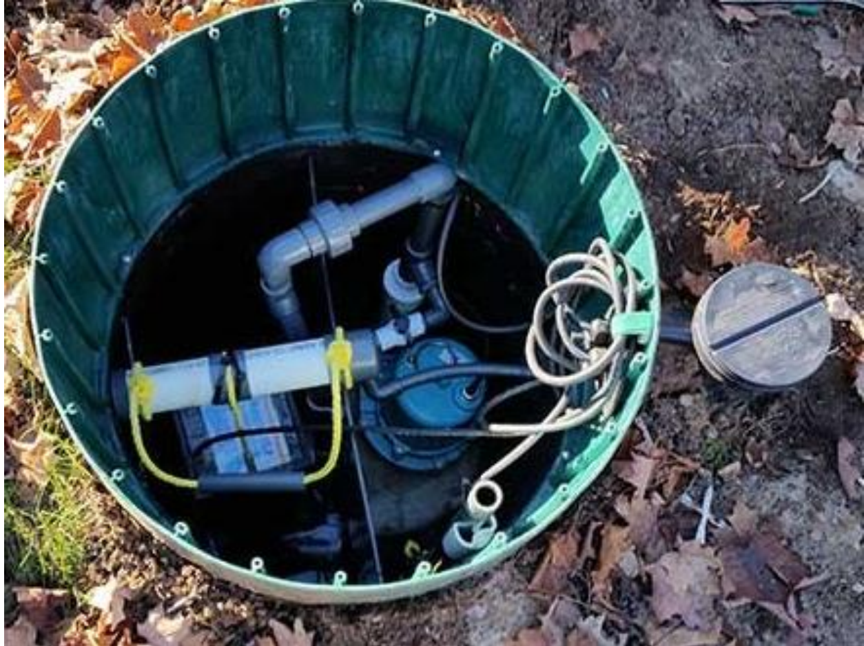
Figure 9. Field installation of Waterloo Biofilter EC-P
