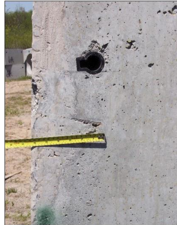
b. Rebar exposed
