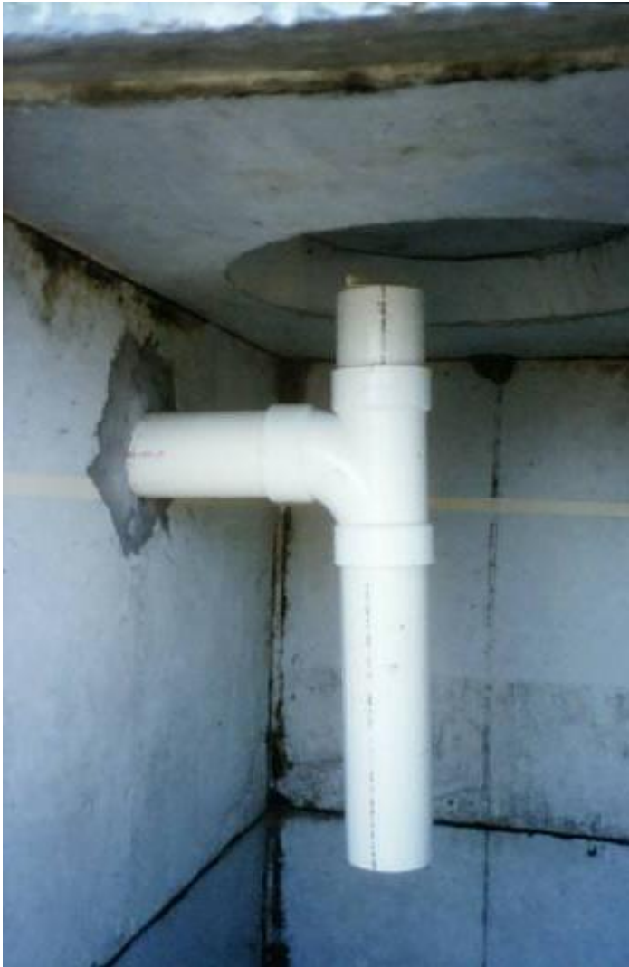
Sanitary on inlet
