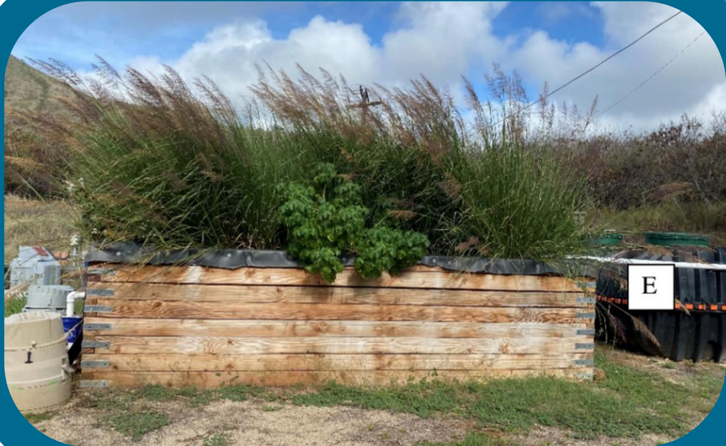
Bioreactor Garden + 1,000 Gallon Septic Tank (Infiltrator IM 1060)
