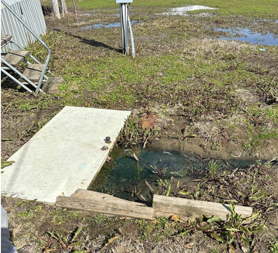
Image: Septic tank without lid, raw sewage on ground
