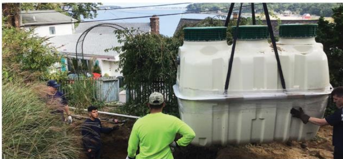
A house in Centerport Harbor gets an enhanced nitrogen removal septic system to replace a cesspool. BIL funding is supporting New York State's effort to replace outdated systems to reduce nitrogen pollution into Long Island Sound. Jim Ammerman/LISS photo
